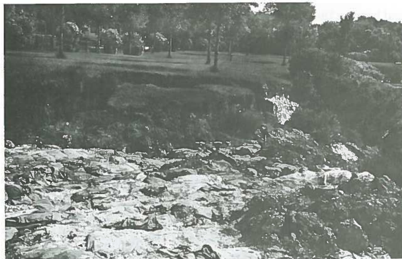
Severe riverbank erosion and sand bag debris at the St. John's Park extension following the 1950 flood. WPRD.
